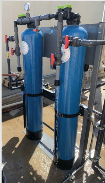
Pump and Treat AFFF-Impacted Groundwater
